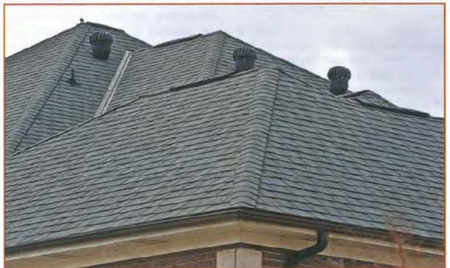
Figure 3 – Example of improper ventilation system using mixed type of exhaust vents on the same attic area. Photo courtesy of Lomanco, Inc.
